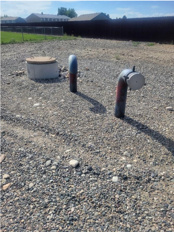
Existing Dry Hydrant
