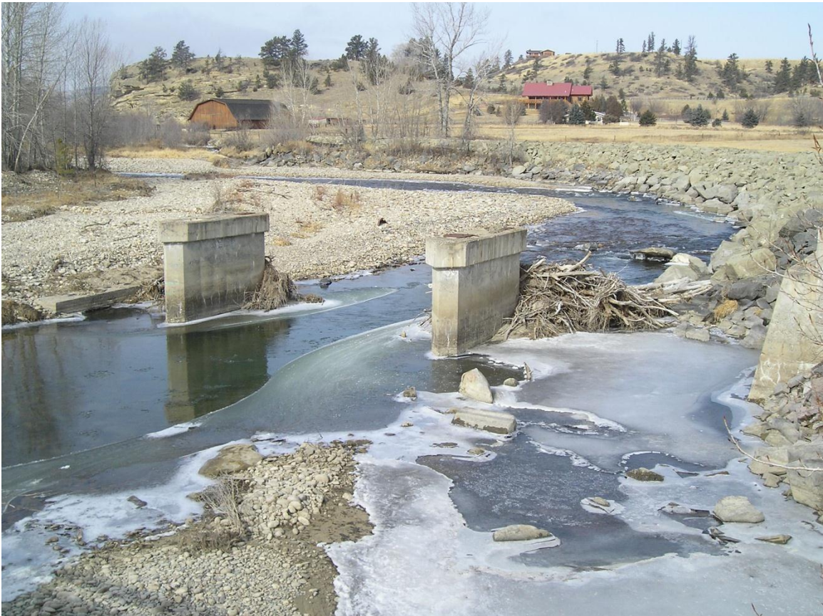
Abandoned concrete piers in Rock Creek upstream of Joliet catch debris. This situation contributed the damaging floods in the spring of 2011. Mitigation 4.1.b would remove these piers.
